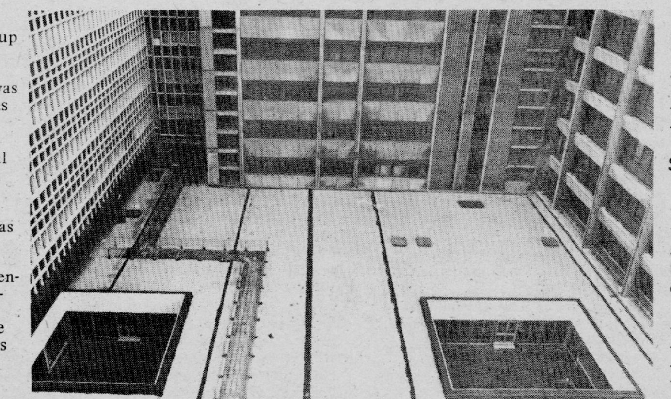
Looking down on to the podium roof. It will have to be replaced because the materials used in the roof are a fire hazard.
