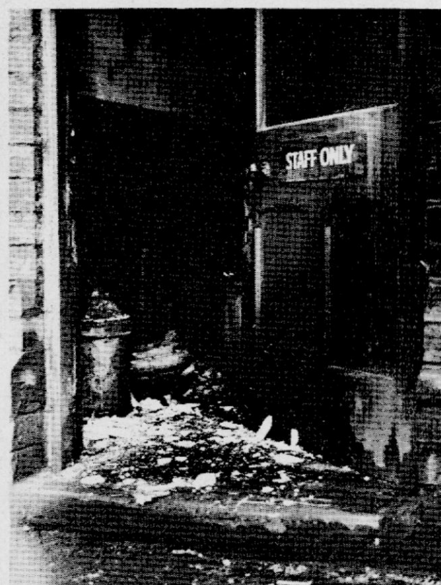
Rubble litters the floor of the former staff room which opens onto the platform at Mersey Road station.
